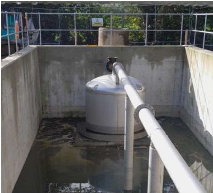
Figure 2: Lifford WwTP CWF Storm Flush Image 1
