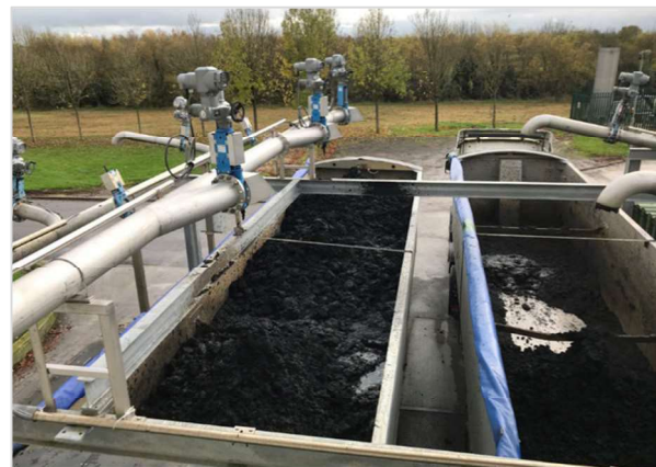
Figure 20: Bunlicky WwTP Dewatered Sludge Storage
