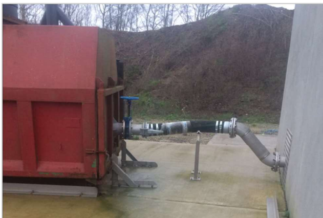
Figure 19: Enniscorty WwTP Dewatered Sludge Storage
